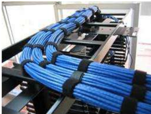
Figura 5.1: Cableado vertical, troncal o backbone
